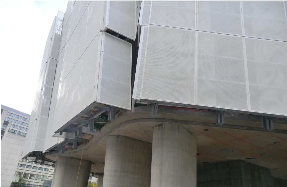
Figure 4: Climbing screen currently in place showing the sloped installation position
