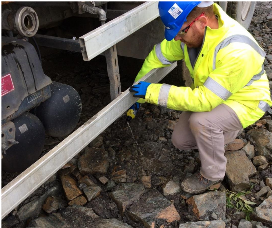
Figure 1 Polysorb being applied to a small oil leak on Tievenameenta Wind Farm
